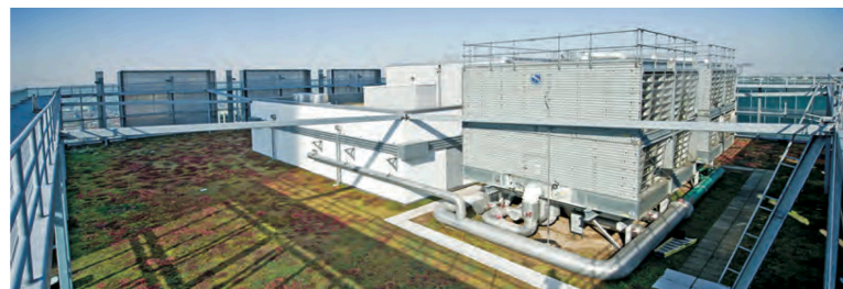
"Green" roof of the 111 South Wacker Drive building, showing planted sedum in the foreground and the building's air conditioning system.
